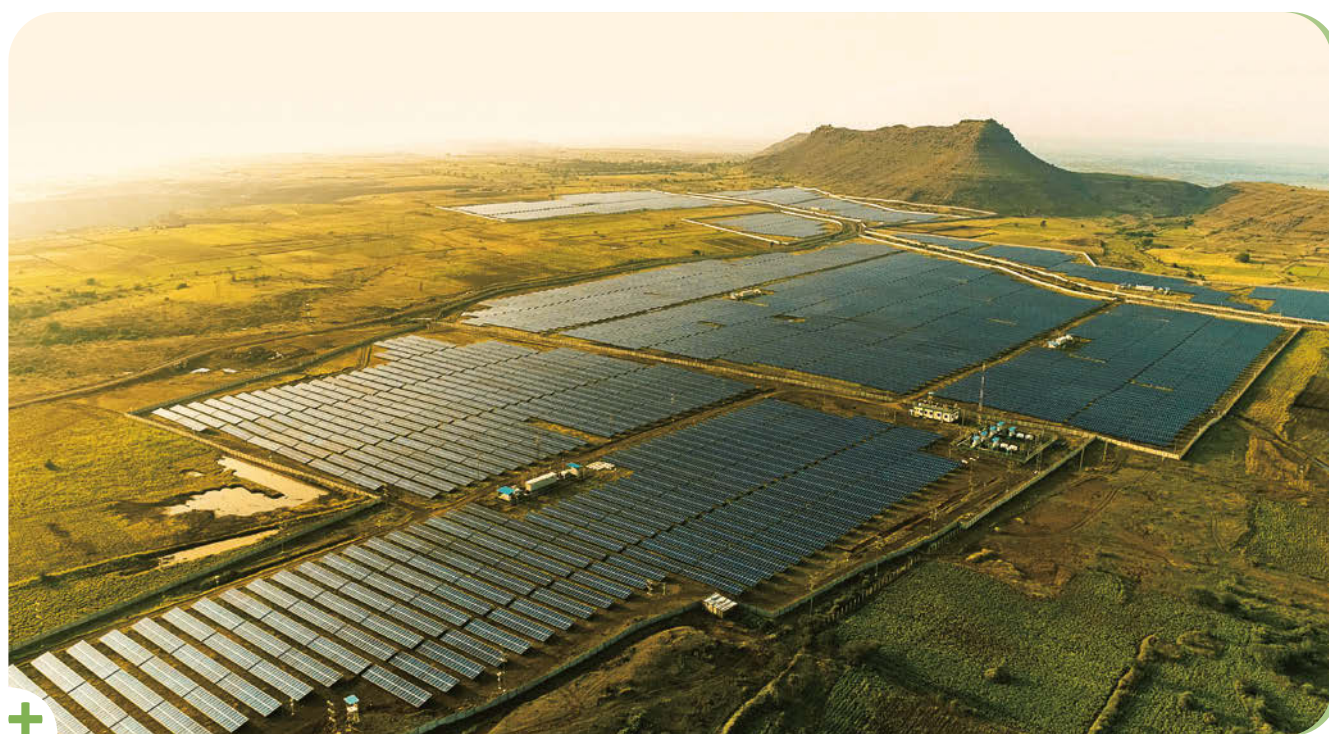
The support of CLP and CDPQ will help accelerate Apraava Energy's growth as a sustainable power company. Pictured here is Gale Solar Farm.
